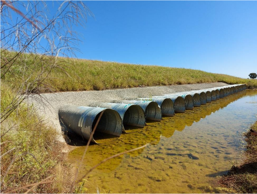
20220726_103111 – Culvert C481 at CH 382.843 - 25 x 1.2m CMP
