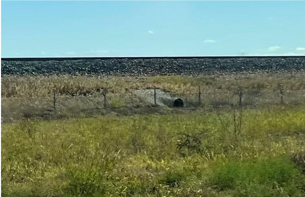
Figure 6-5 Fauna connectivity structure – snake fencing and under track tunnel (every 100m in some locations)
